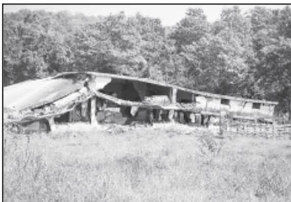
School building at Maitha in Konta tahsil blasted by the Maoists
